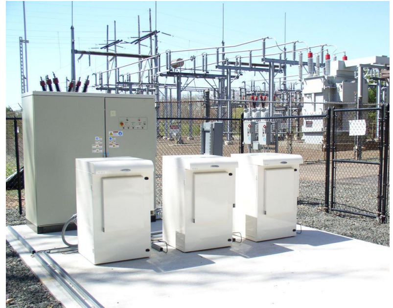
Electric Utility Substation
