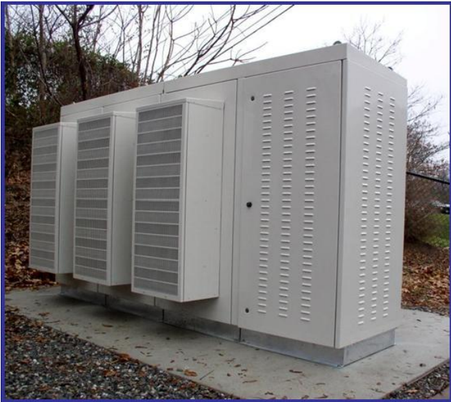
Telecom Switching Station
